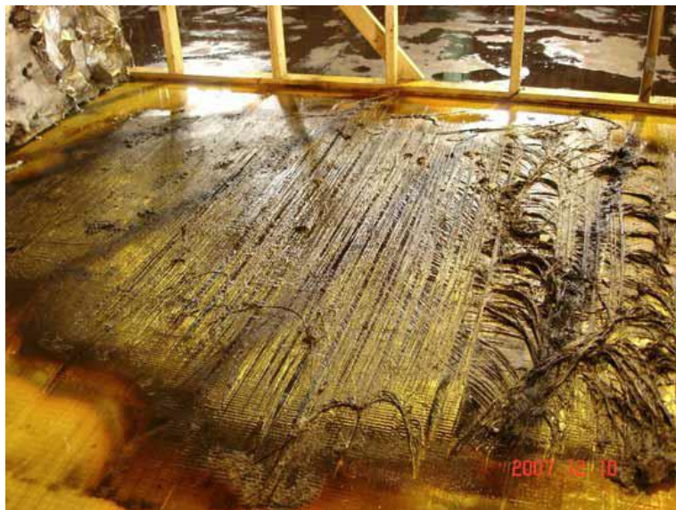
Figure 4.6. Damages to the FRP composite deck as a result of the uncontrolled fire, after the floor construction had been removed.
